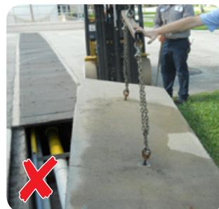
Dangerous lifting technique without Fibrelite lifting aid.
